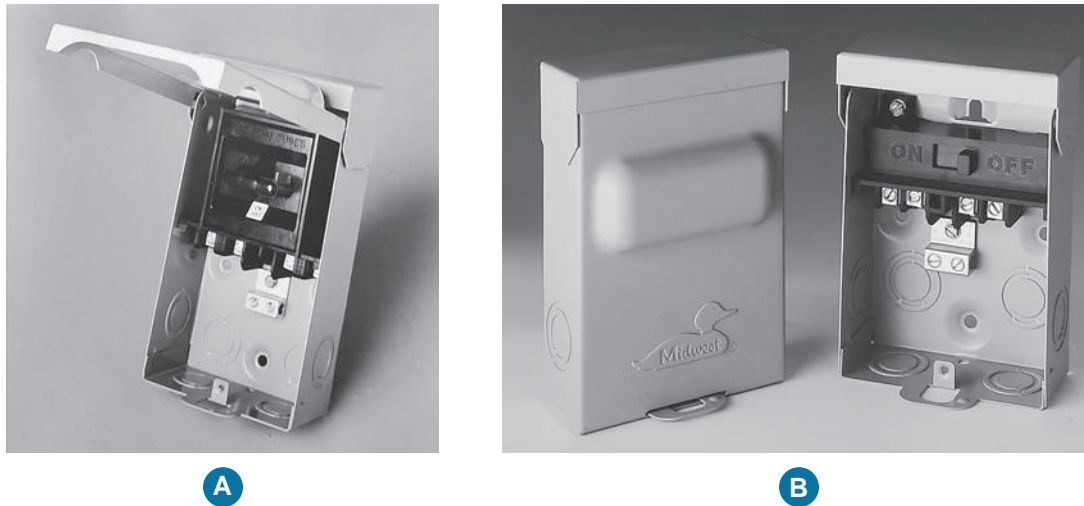
FIGURE 23-21 (A) is a pull-out fusible disconnect. Fuses are inserted into fuse clips on the pull-out device. Insert the pull-out device for “On,” and remove the pull-out device for “Off.” (B) is a nonfusible disconnect, available in 30- and 60-ampere ratings at 240 volts. Both have padlock provisions to prevent unauthorized tampering. Air-conditioner disconnects are available that have a GFCI receptacle as part of the disconnect enclosure. The GFCI receptacle must be wired to a separate 20-ampere, 120-volt branch circuit. (Courtesy of Midwest Electric Products)
