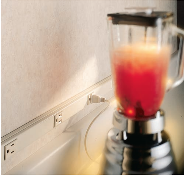
FIGURE 18-19 A multioutlet assembly installed above the backsplash of a kitchen countertop. (Courtesy of The Wiremold Company)
