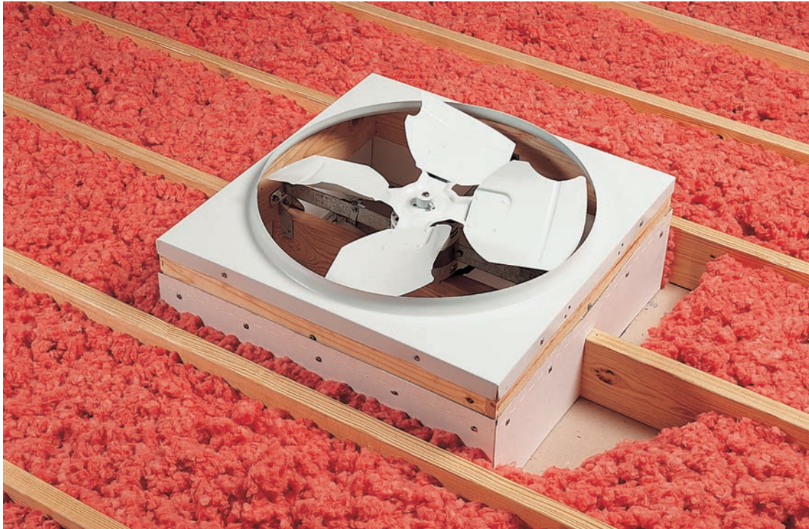
FIGURE 22-4 Ceiling exhaust fan as viewed from the attic. (Courtesy of Broan-NuTone)
