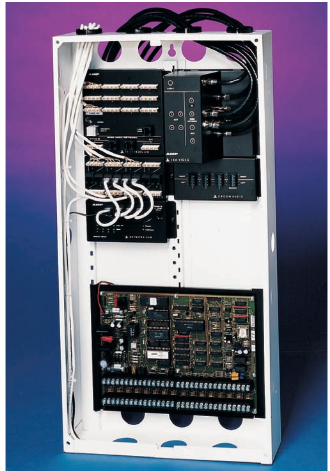
FIGURE 31-6 A “service-center” is the hub of a structured wiring system with telecommunications, audio, video, and home automation controllers installed. (Courtesy Leviton)
